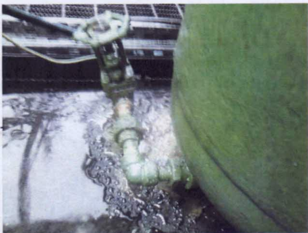
FIG. A: THREE QUARTER PIPE THAT SPILLED OIL
