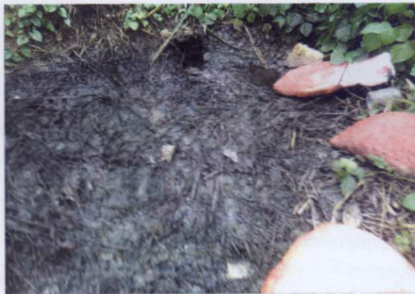
FIG. C: TREATED WATER DISCHARGE PIPE OPENING
