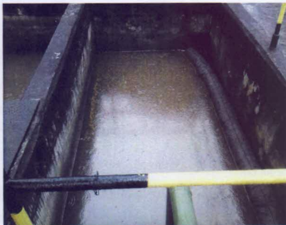
FIG. B: THE SERVER PIT ROM WHERE OIL ESCAPED
